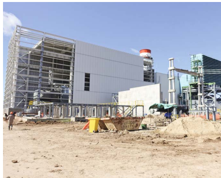
Combined cycle power station in Argentina
