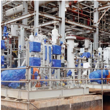
Preservation measures in a refinery
