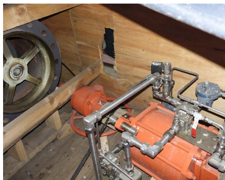
Insufficient and faulty preservation measures
