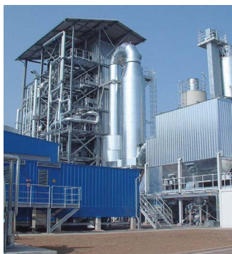
PARTIAL VIEW OF A BIOMASS POWER PLANT
